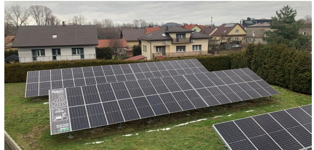
Photovoltaic installation at the Okocim Brewery in Brzesko.
